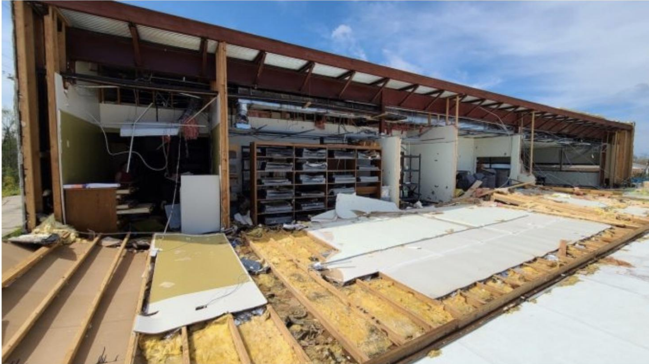
The second floor of the West Regional Library in Luling sustained significant damage in Hurricane Ida.
